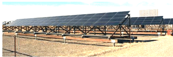
Photo 1. Fields of PV (Photo Courtesy of NREL).
